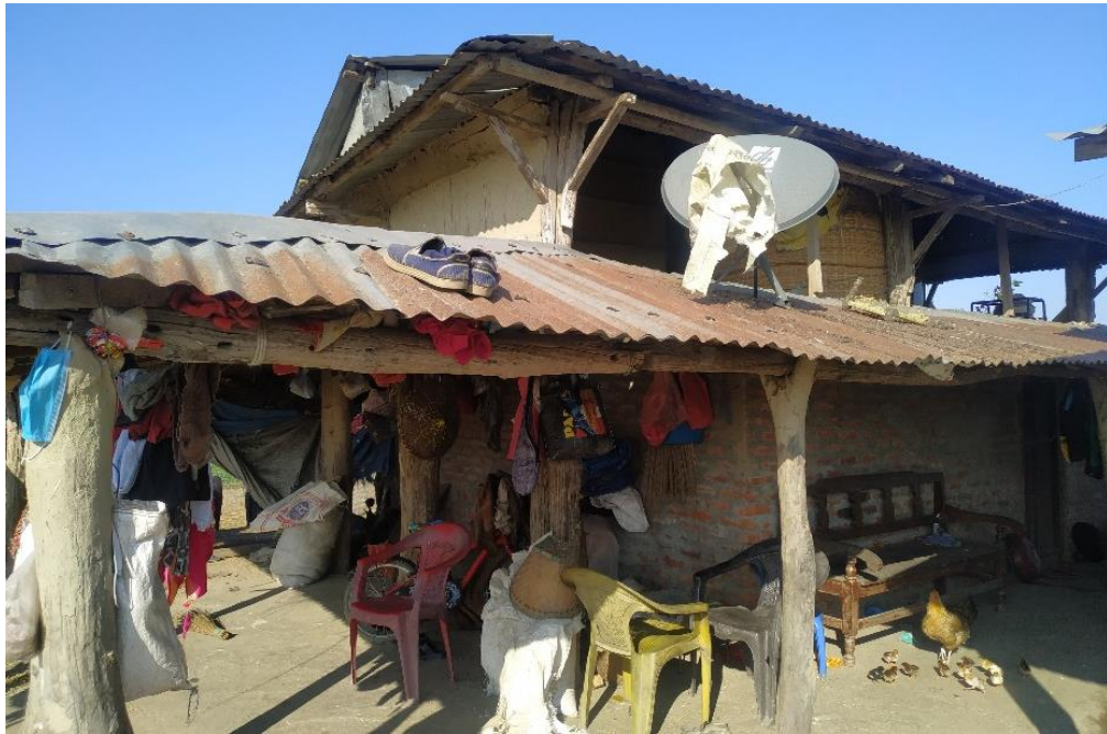
Figure 8: The house which was relocated to different places, still had the same old timber structural elements. The house was intervened with brick masonry wall and the inside is used for kitchen. Upper floor is used for granary storage.
