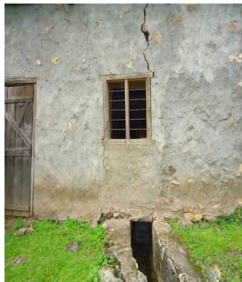
Power House of MHP of Cherranga Khola(Kotdurbar)
