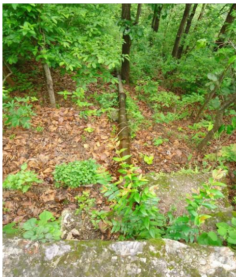
Penstock pipe of Kota Barsha Khola MHP
